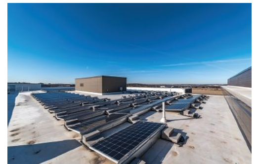
On the exterior of the building, this VRF system requires no unsightly rooftop units and screening.
